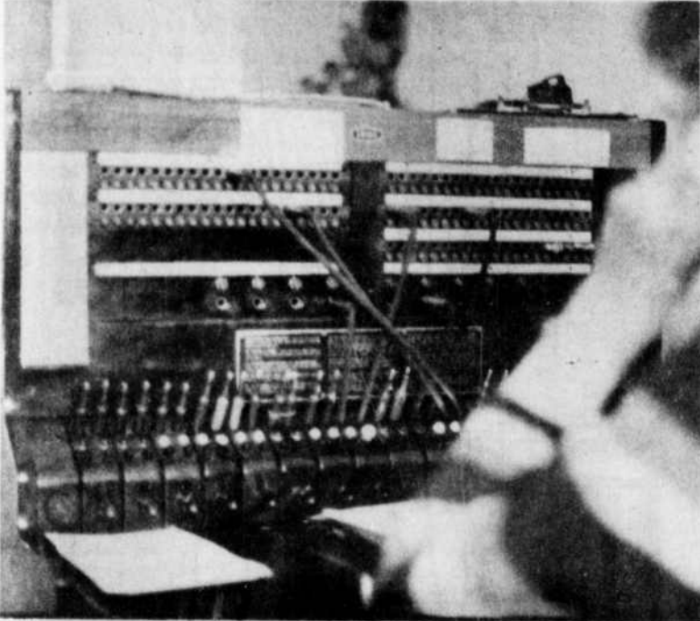
The present 26 year-old switchboard in Roberts Hall will soon be replaced by a newer model. (Photo by Edythe Mentasana)
